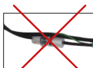
Water trap NOT OK
