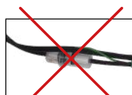
Water trap NOT OK
